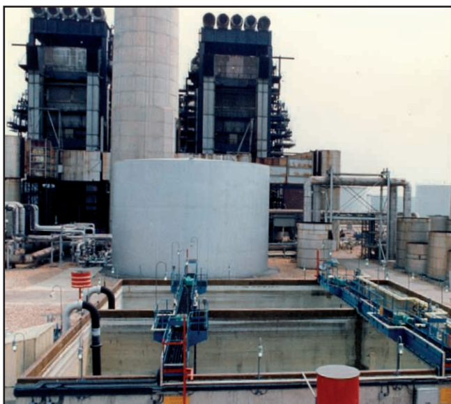
Tanks lined with 600 Series lining at effluent treatment plant.
