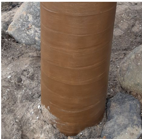
The Denso SeaShield Series 70™ System as used on the Cornwallis Wharf in Auckland.
