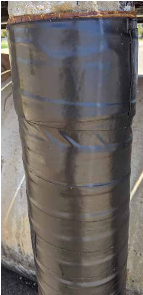
The Denso SeaShield 80 system used on the Shelley Beach Park Recreational Jetty.
