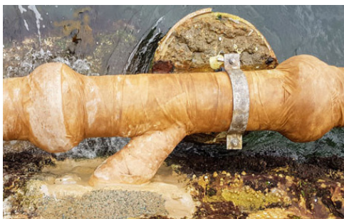
The Denso SeaShield 70™ system used to protect pipe and flange connections on the Kirribilli Aqueduct in Sydney Harbour.
