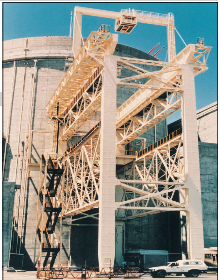
▲ Fig 1. Steelcoat 400 protects all areas, including hand rails, of badly rusted / pitted gantry crane situated in a nuclear power plant. Conventional paint coating failed after only 4 years service.
