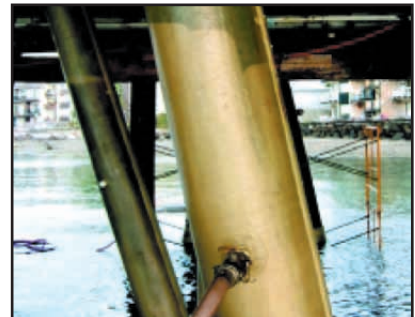
Pumping the Grout into the GRP Form. (note the visible rising grout level seen through the Form).
