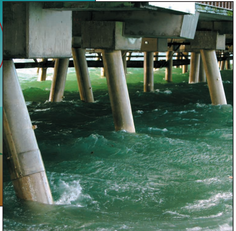
Above: A completed SeaShield Series 500 system in service.
