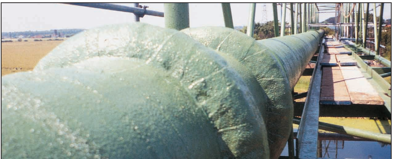
Exposed pipe and pipebridge: Profiling Mastic has been utilised at the flange areas to provide a profile for tape application.
