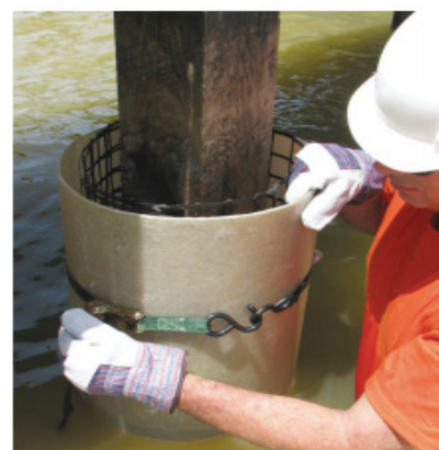
Figure 4. ▲ Grout can be pumped as soon as the Fiber-Form Jacket is secured
