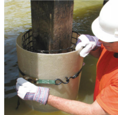
Figure 4. Grout can be pumped as soon as the Fiber-Form Jacket is secured
