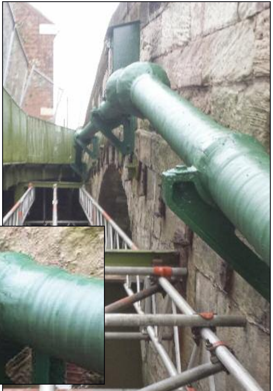
The Rocester Pipebridge protected with a combination of the Denso Steelcoat 100/400/700 Systems
