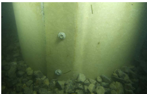
The Denso SeaShield 70™ & SeaShield 400™ Systems as used on the Station Pier pile rehabilitation works.
