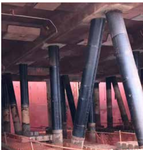
The Denso SeaShield 2000FD system used on the BHP Wharf Remediation Project.
