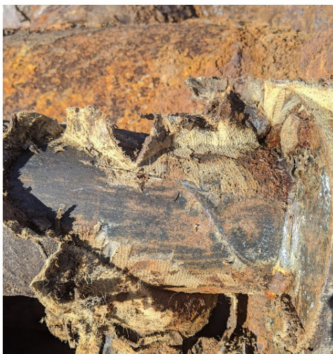
Water main wrapped in Denso™ Tape more than 50 years ago.
