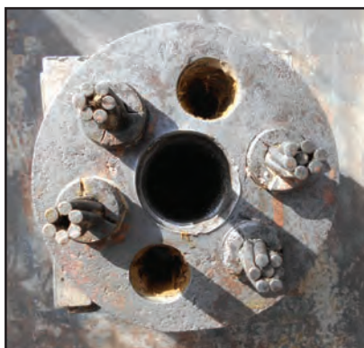
Top: Condition of the original Denso Covercoat System protecting the anchor heads, without any maintenance, after 25 years in service.
