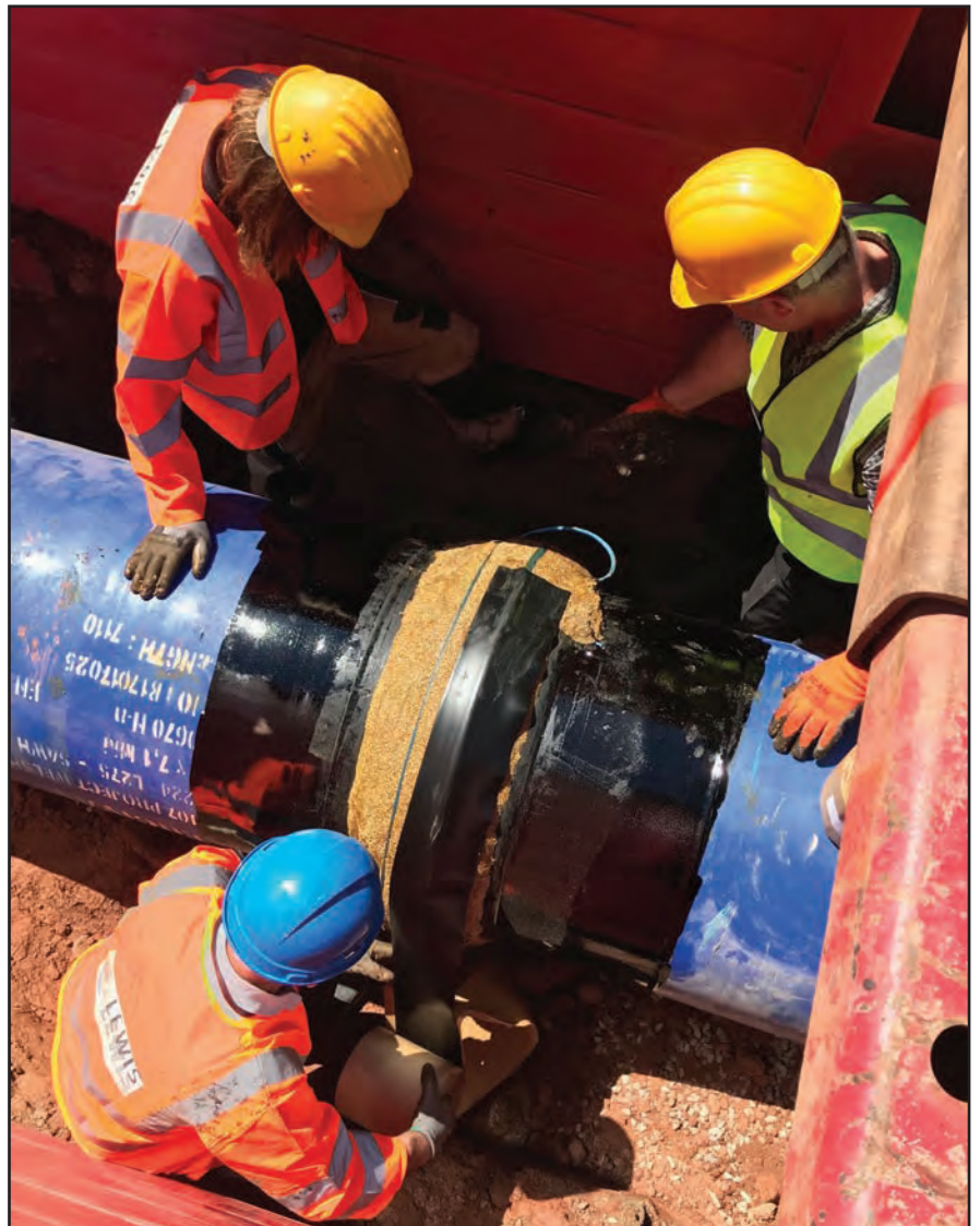
Winn & Coales (Denso) Ltd Area Manager, top right, trained Lewis Civil Engineering staff to achieve the best application of the Denso P2 Joint Protection System.
