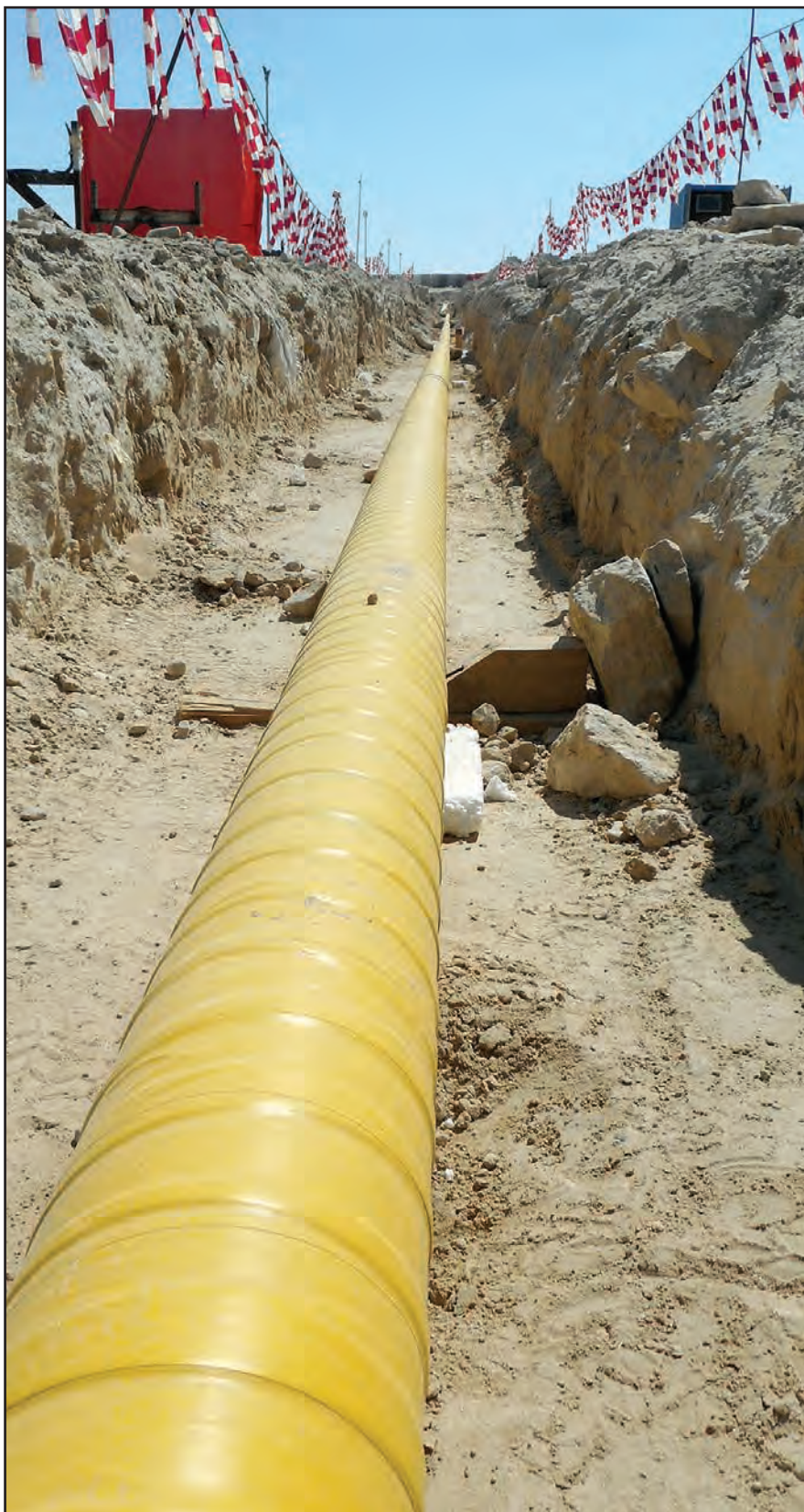
Picture of the completed second system for larger diameter pipes prior to backfill.
