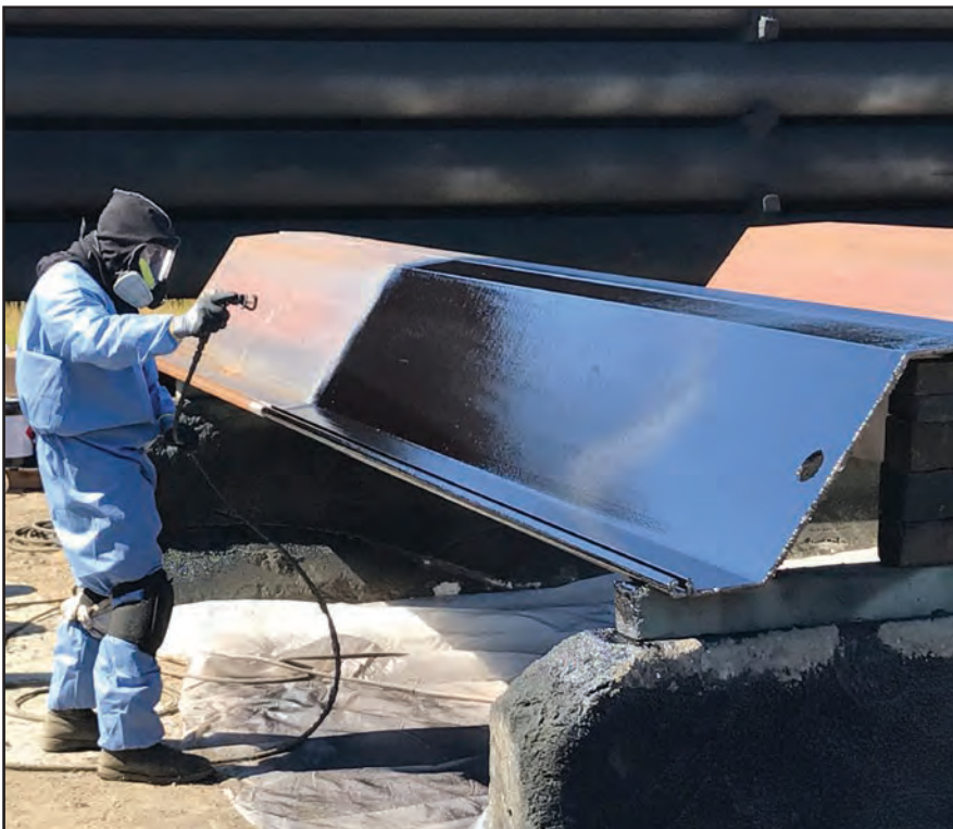
Above: Application of Protal 600 CTE using a single leg airless spray pump.
