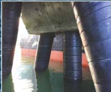
SeaShield System protecting wood pellet export facility support piles - Canada.
