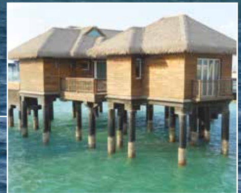
SeaShield System protecting holiday villa support piles - Qatar.
