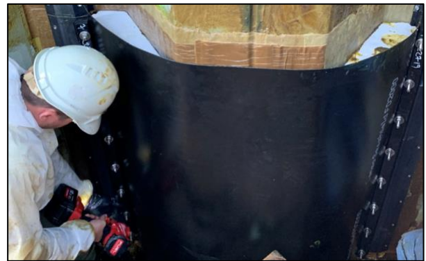
Figure 2. (1) Installation of the system; (2) note the petrolatum tape and rigid foam; (3) the worker is tensioning the outer covering.
