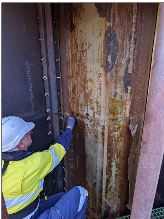
Figure 4. (1) Inspection of a trial after 2 years; (2) the outer covering, foam blocks and petrolatum tape have been removed for inspection of the steel surface; and (3) the petrolatum primer is still in place on the steel surface and water ingress has not occurred.
