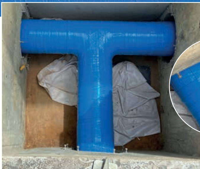
Above: Viscowrap™ HT applied to a tee junction. Centre: The completed Viscotaq coating is checked for holidays. Right: A wrap of black Denso PVC Tape completes the protection.
