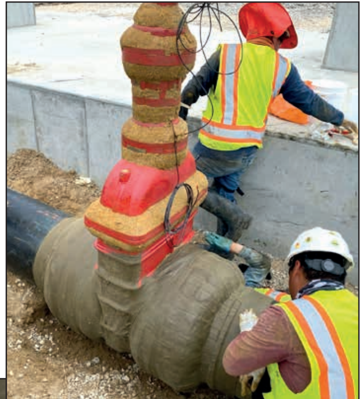
Large water valve completely encapsulated with the Denso Petrolatum Tape System will provide decades of corrosion prevention.
