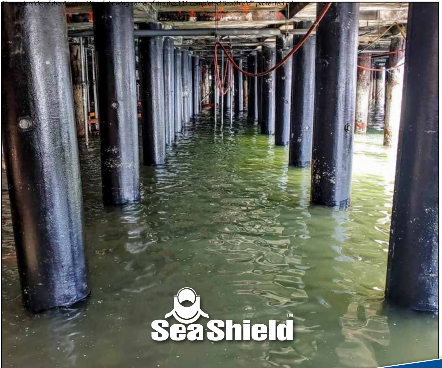
The underside of the Alcatraz Wharf showing some of the the 111 completed SeaShield™ protected piles.
