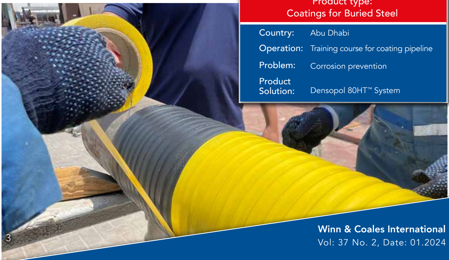
Below: Denso PVC SA Tape™ is then applied to the pipe lengths over the DensoPol 80HT™ for extra mechanical protection during transportation.
