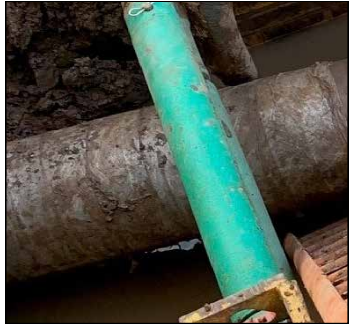
View of pipe after it had been pulled under the roadway. Denso Bore-Wrap™ is still intact so there is no damage to the pipe coating.
