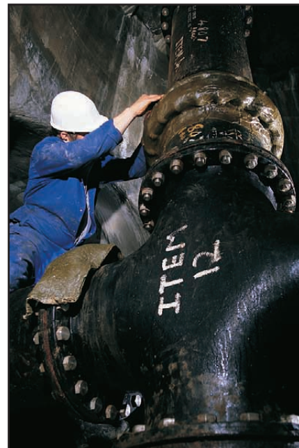
Sealing and wrapping flanges on damp pipes in a continuously humid environment.
